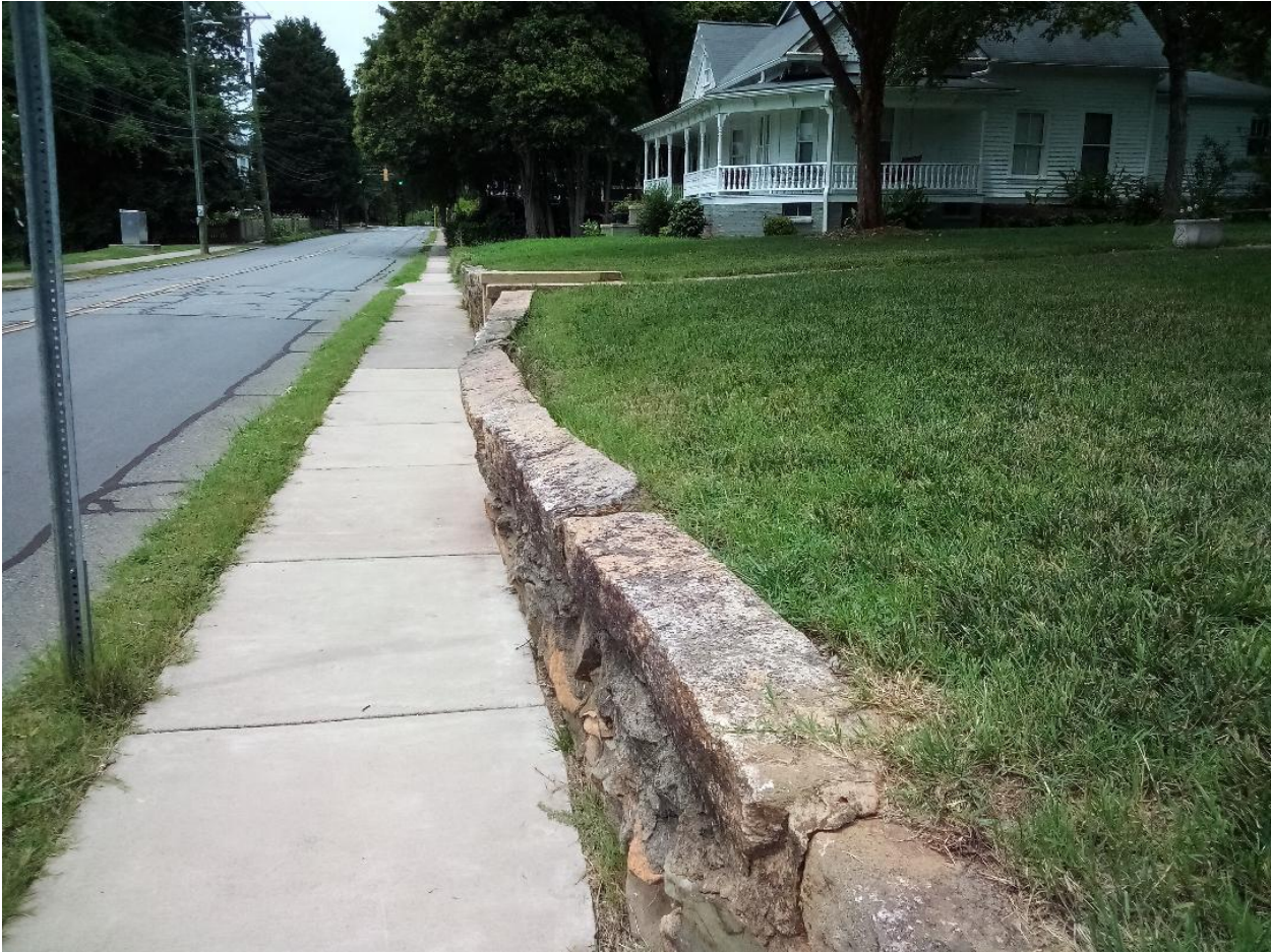
H-19-22 Existing Masonry Retaining Wall – Bowing on Right Side
